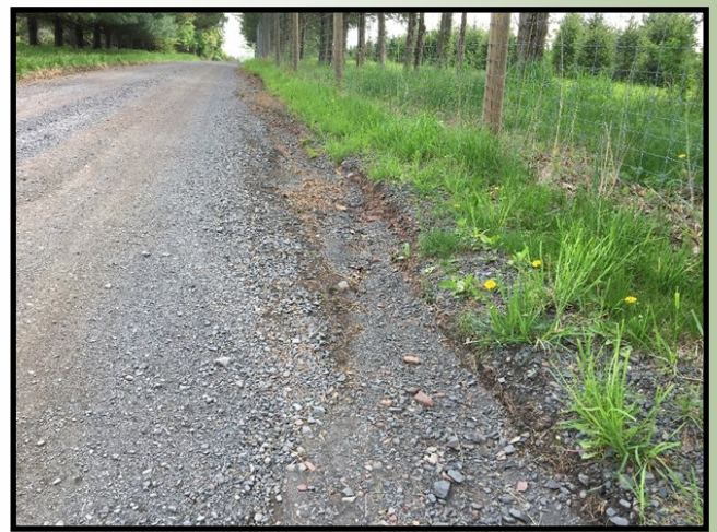
Large amount of sediment traveling in the ditches before proposed improvements
