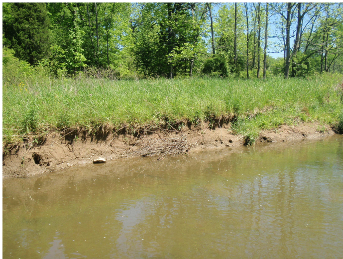
Problem Area – PD3
