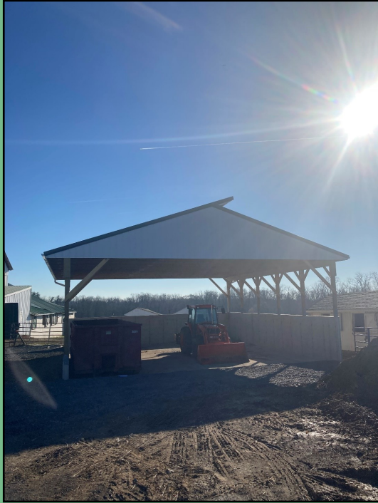
Above: Photo of a manure storage facility completed in the Fall of 2022 for an equine farm. This was built as part of the Growing Greener grant mentioned previously.
